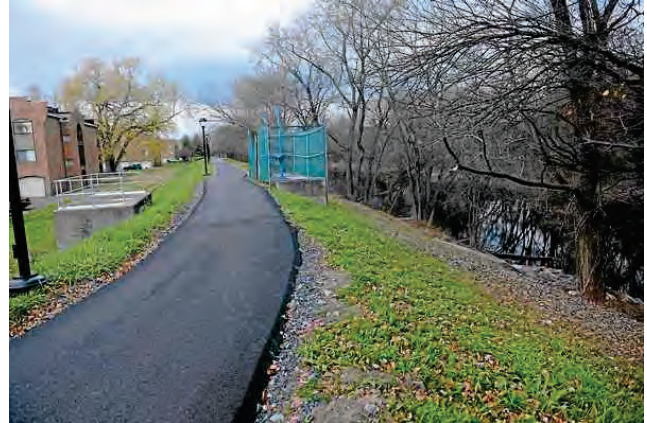
A look at the levee dividing Esopus Creek and the Dutch Village apartments in Kingston 17
