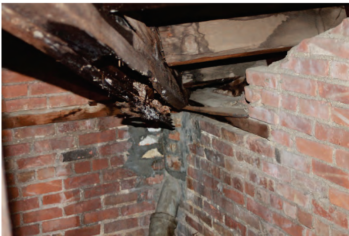
Interior and exterior building damage
