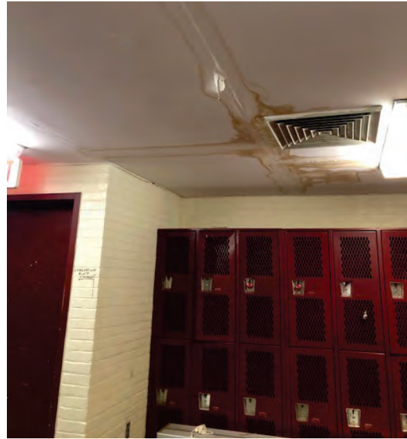
Locker room conditions
